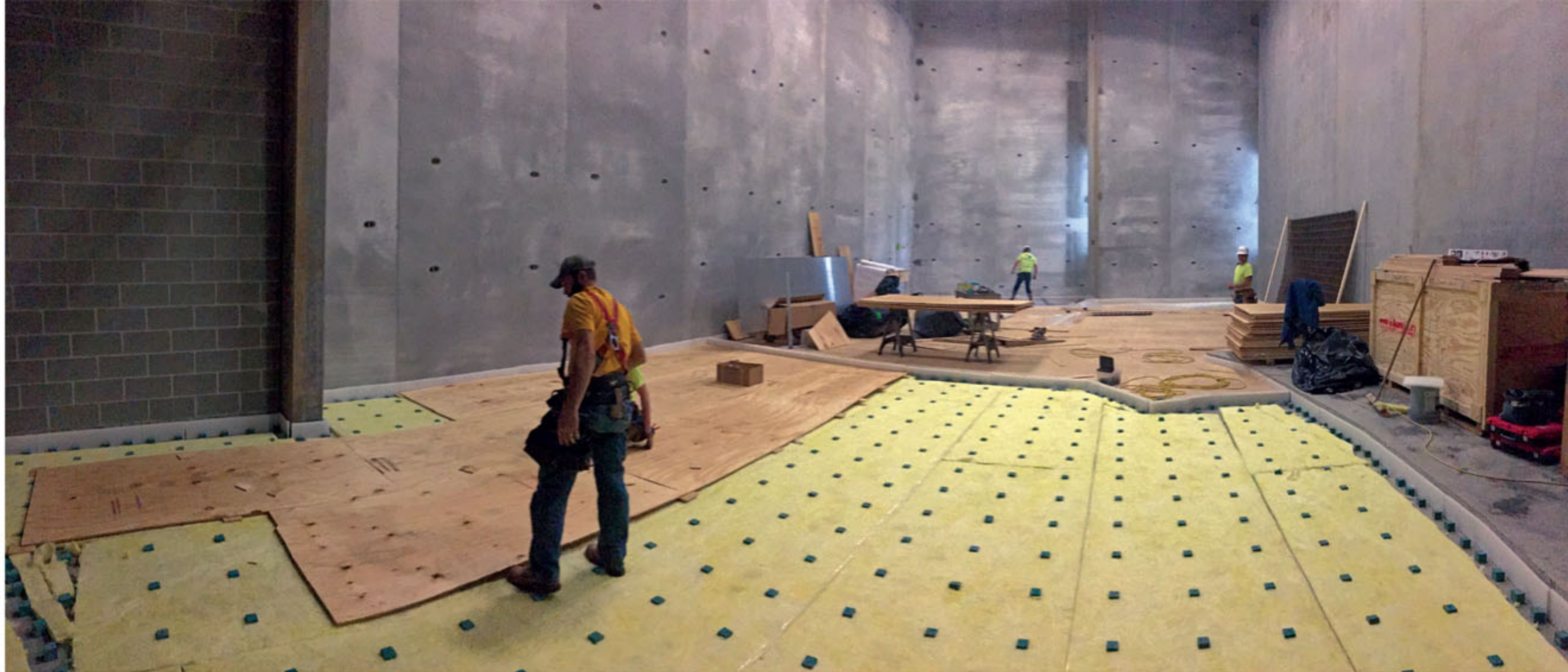
The room layout begins to take shape as the floating floors are laid down.
